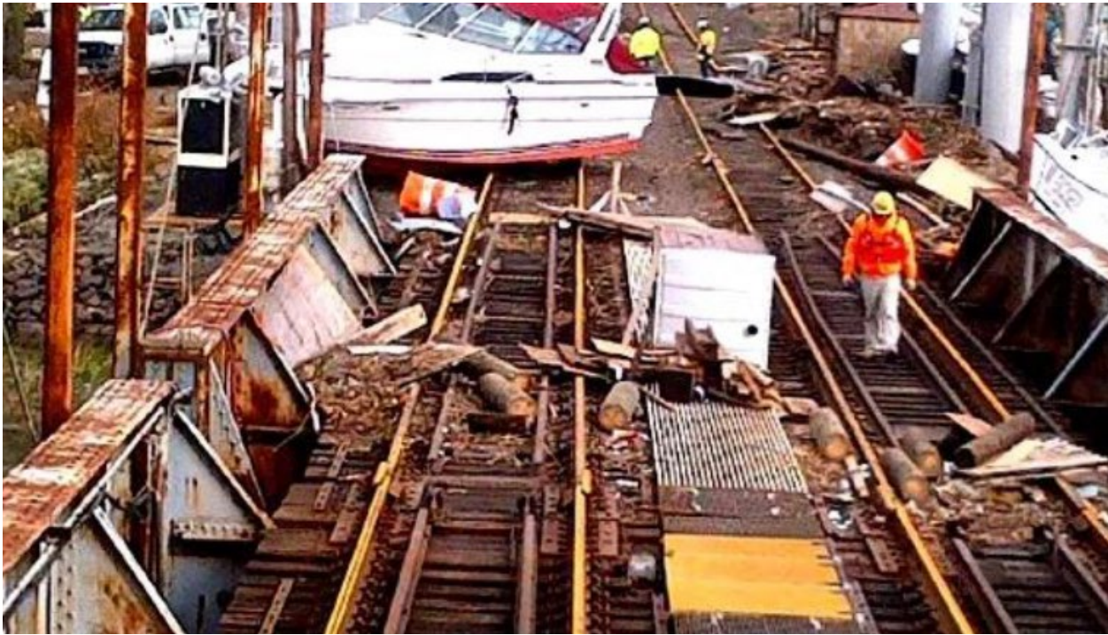
Figure 2. Track Damage in Queens After Hurricane Sandy
