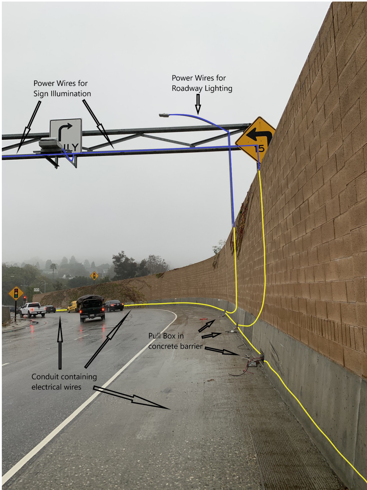
Figure 1. Illustration of Copper Wire Use in Roadways -- Northbound Route 405 Sunset Blvd Off-Ramp. Yellow and blue lines represent copper wire in the infrastructure.
