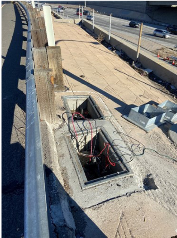
Figure 3. Two vandalized tamper resistant pull boxes at Branford St. on-ramp to Southbound CA I-5 Fwy.
