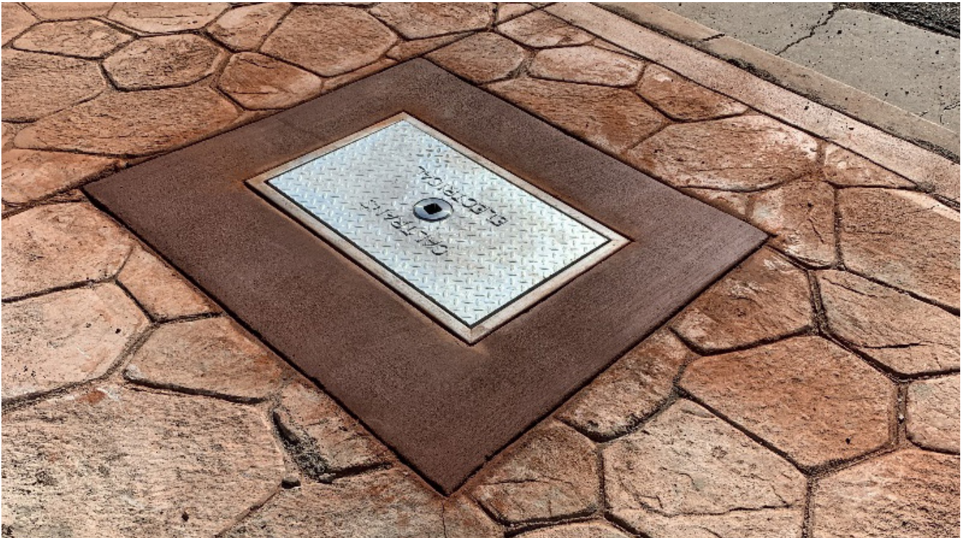
Figure 5. Latest tamper resistant pull box that requires proprietary tool to open, located at southbound Pearblossom Hwy to southbound CA-14 Hwy gore area.
