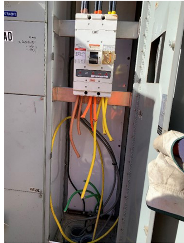
Figure 4. Vandalized emergency power feeder at CA I-5 Fwy., Southbound CA-14 truck lane tunnels.
