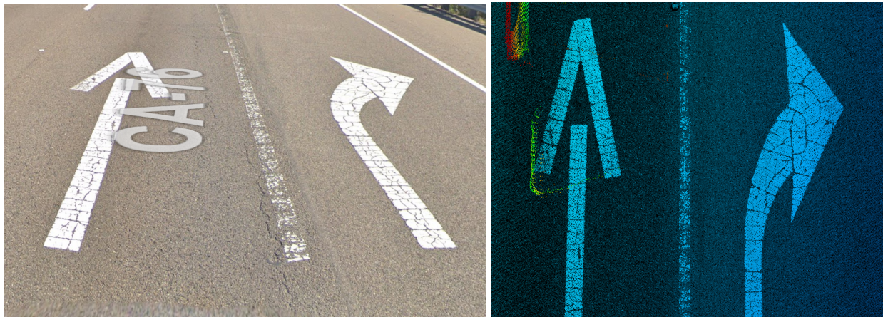
Figure 4. Example of the Road Condition on Road Marks in the Google Street Map (Left) and MTLs Point Cloud Data
