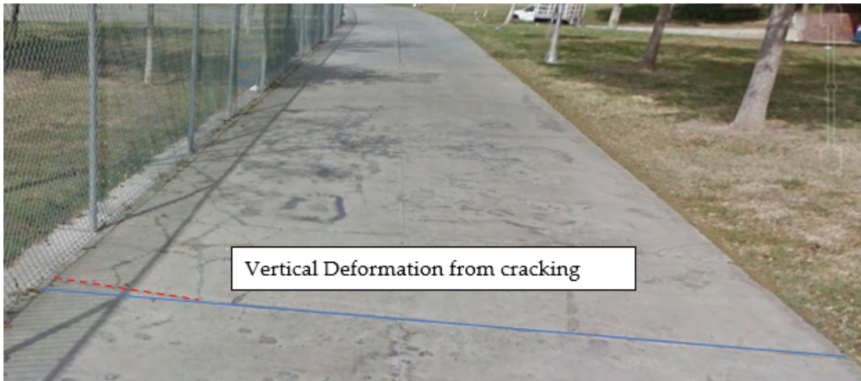
Figure 8. Site #3 Concrete Pavement - Cracking, Joint Deterioration, Roughness, Surface Defects
