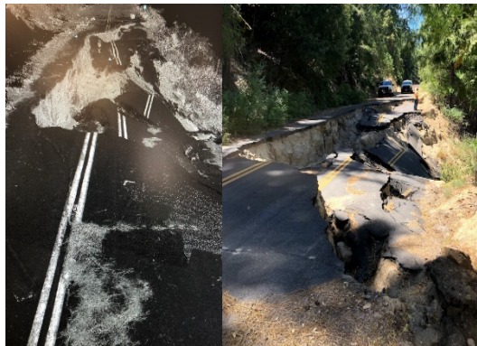
Figure 3. Terrestrial LiDAR Scan and Photo of Failed Pavement
