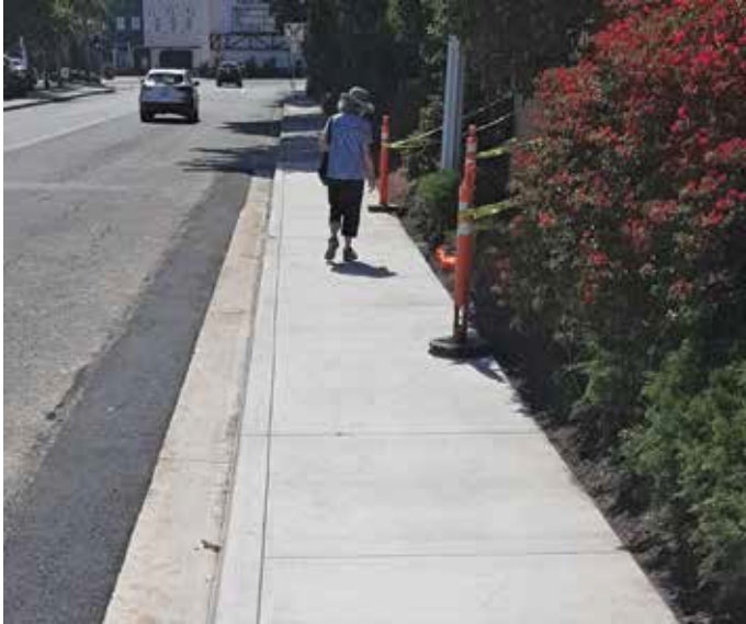
New sidewalk on east side of Fairview Avenue, due to work of Encina Royale residents.
